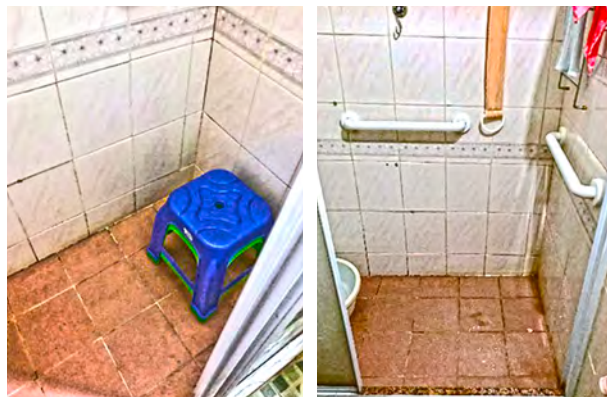
Fig 7 and 8. Before (left) and After (right) home environment modification with rail installed
