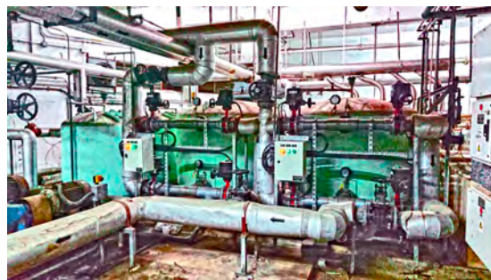
Fig 2. The water plant for running the hydrotherapy pool in the MacLehose Medical Rehabilitation Centre
